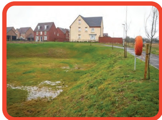
SuD design with little consideration and ecological value does not contribute to placemaking and creates potential trip hazards
